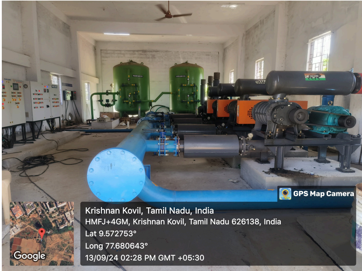
Air Blower Pumps Facility in the STP at Kalasalingam Academy of Research and Education
