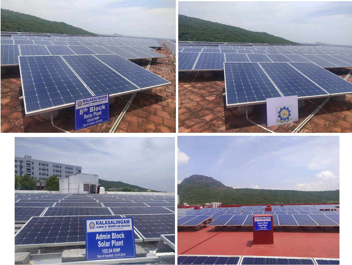
Solar Plant in KARE Campus
