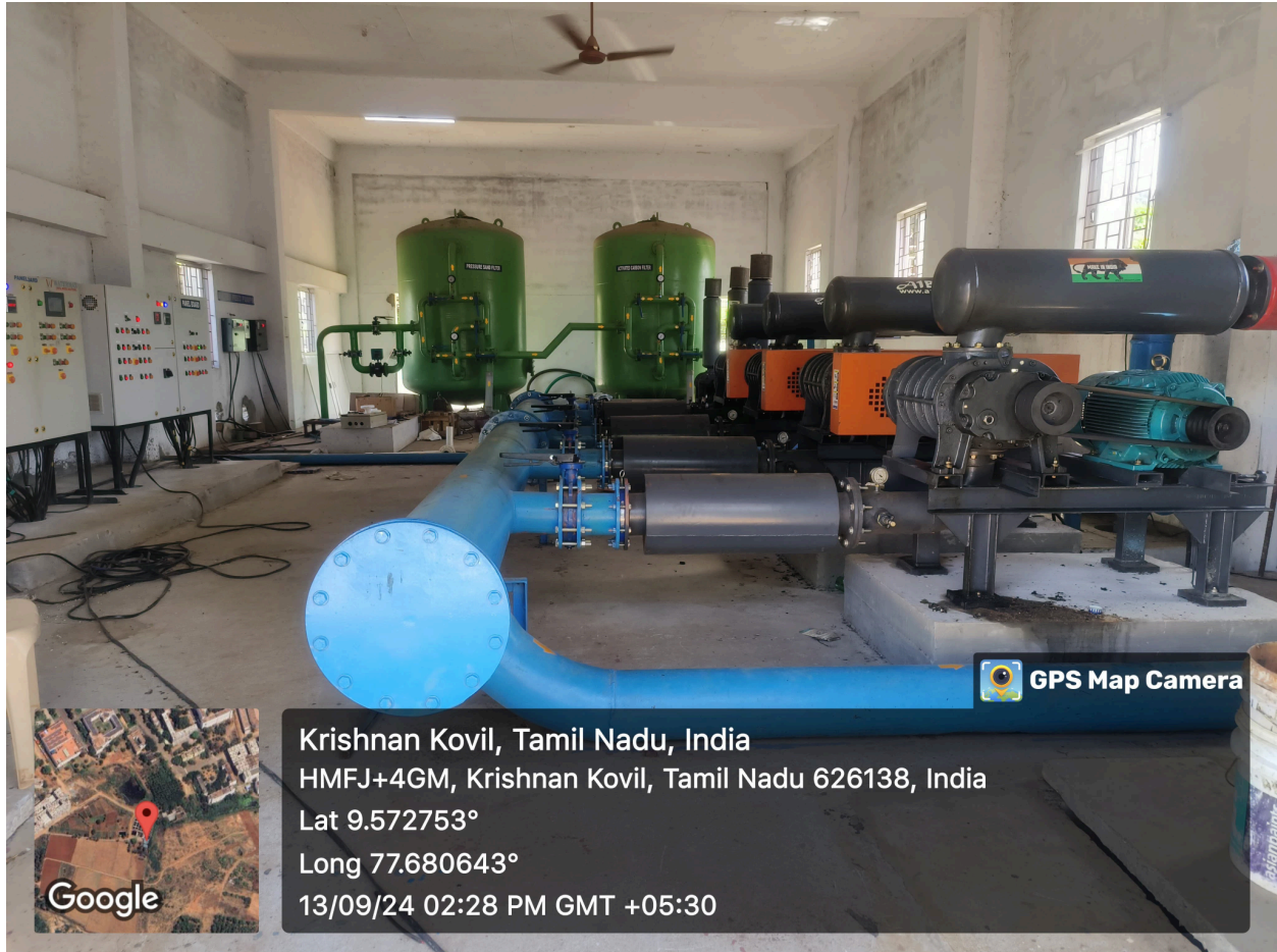
Air Blower Pumps Facility in the STP at Kalasalingam Academy of Research and Education, TN
