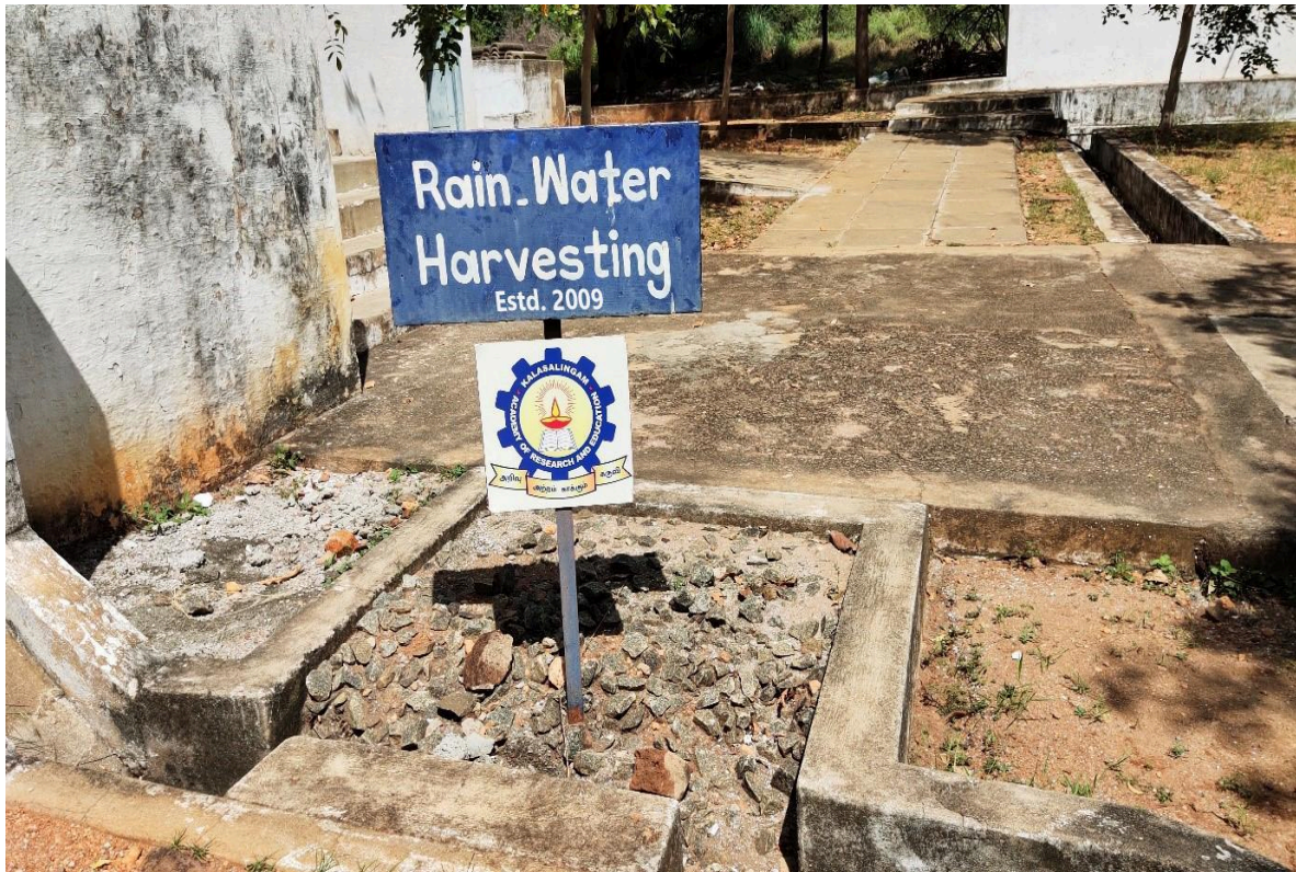
Rainwater Harvesting System near Homi. J. Bhabha Block / Block-II / Chemistry Lab
