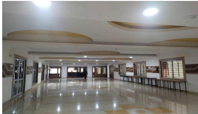
LED lights installed in all building
