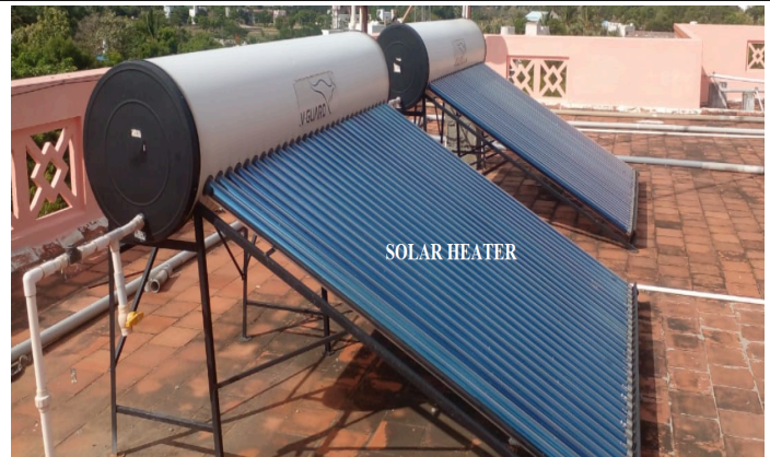
Solar Water Heater (Close view)
