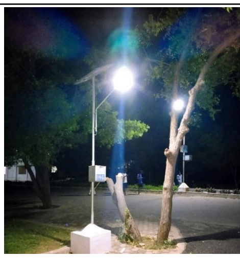
Solar street lighting (Single pole view)
