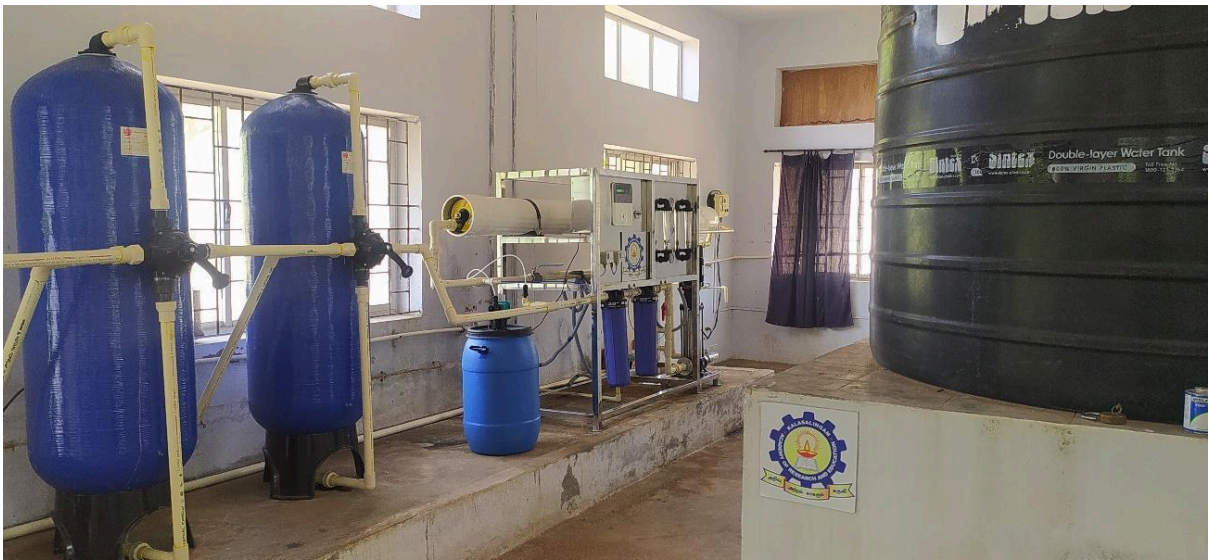
Reverse Osmosis plant
