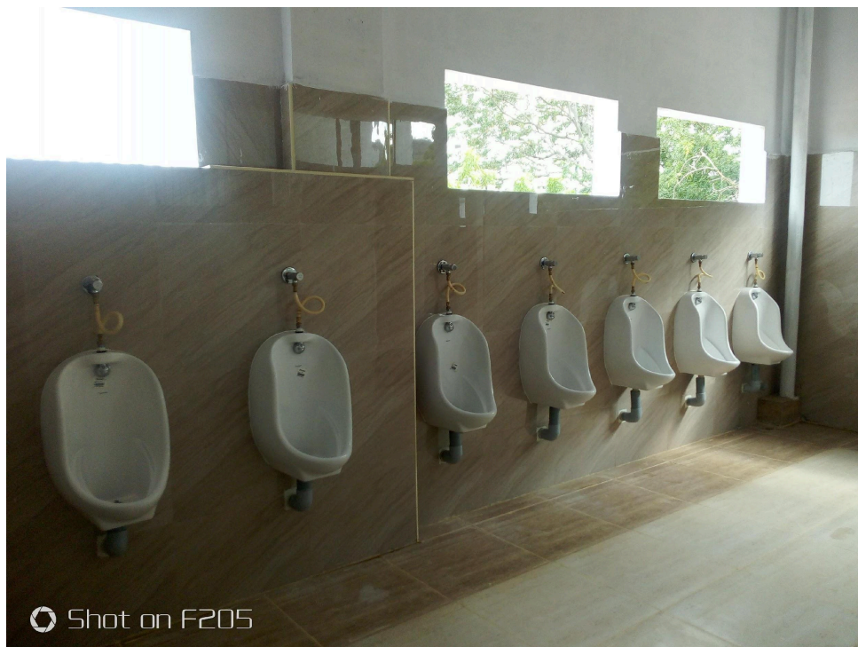
Recycled water used for flushing of toilets
