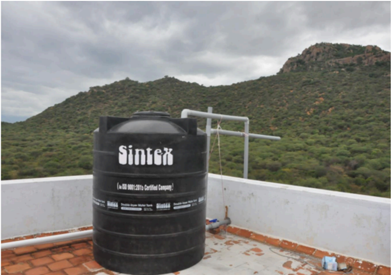
Figure:2 Dual Pipeline system used for treated water
