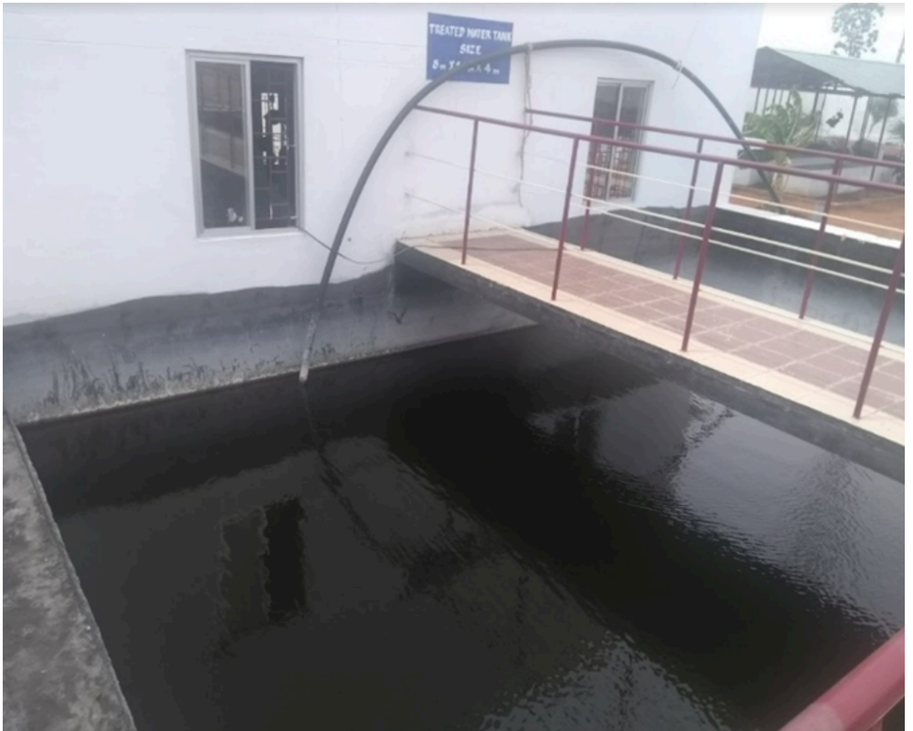
Figure 9: Storage Tank for Treated Water
