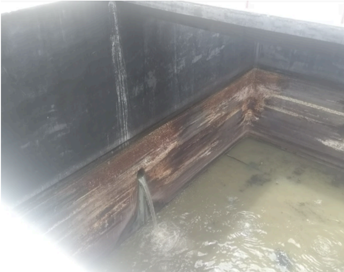
Figure 3: Wastewater Collection Tank (5 KLD)
