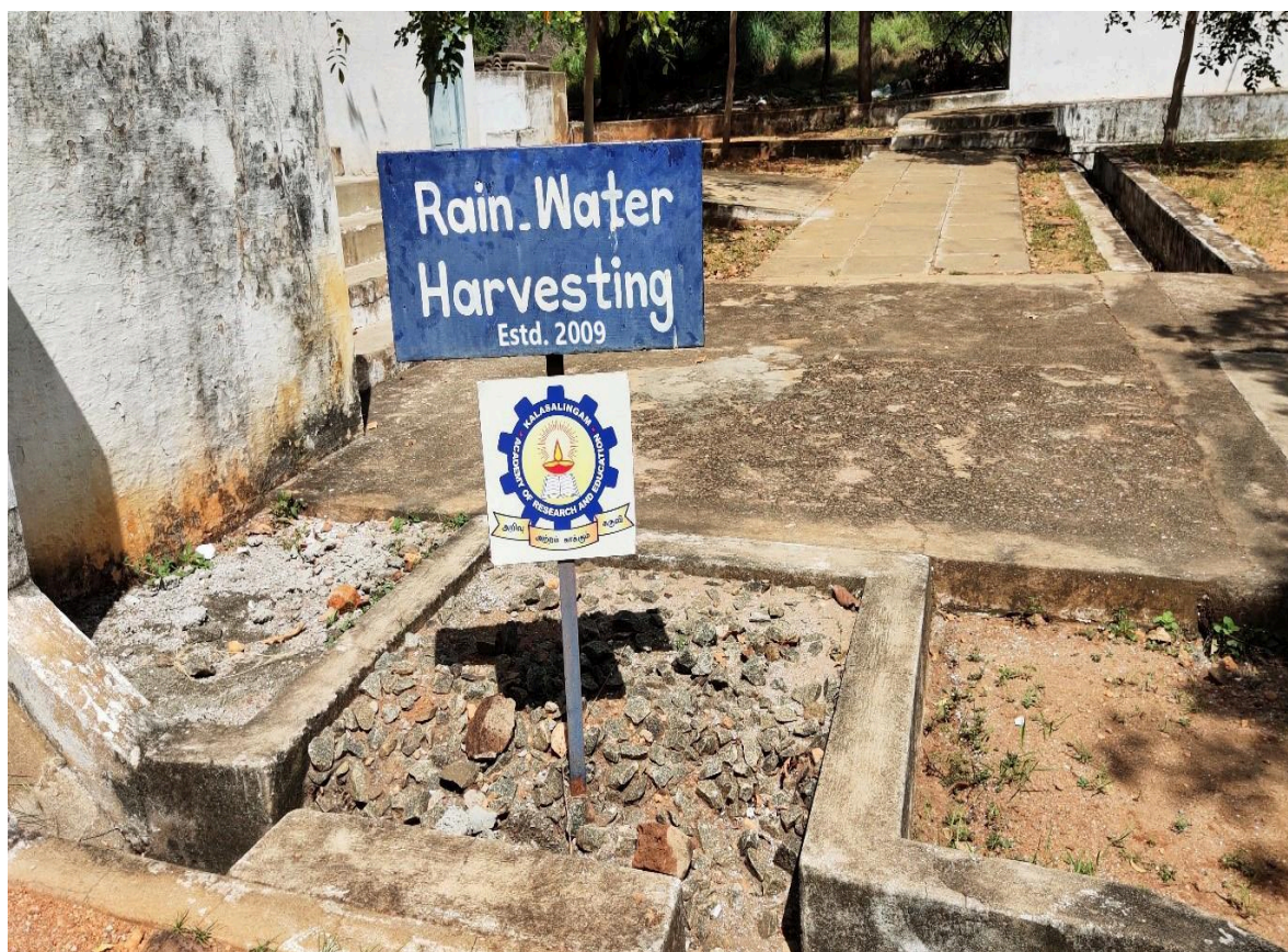
Rainwater Harvesting System near Homi. J. Bhabha Block / Block-II / Chemistry Lab
