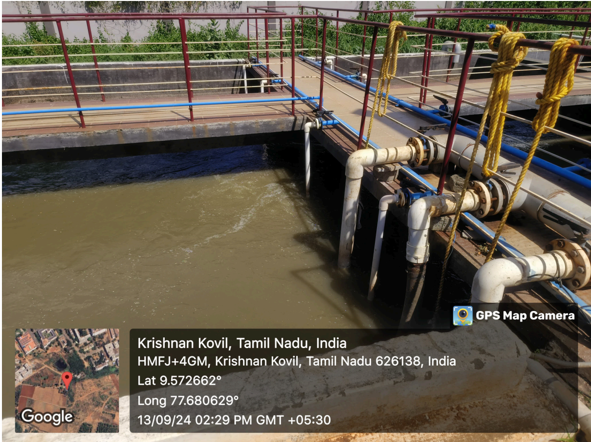
Aeration Tank Facility in the STP at Kalasalingam Academy of Research and Education, TN
