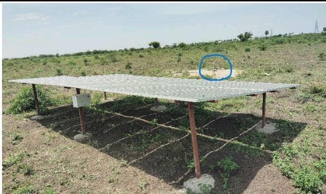
Solar Water Pumps
