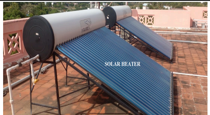
Solar Water Heater (Close view)
